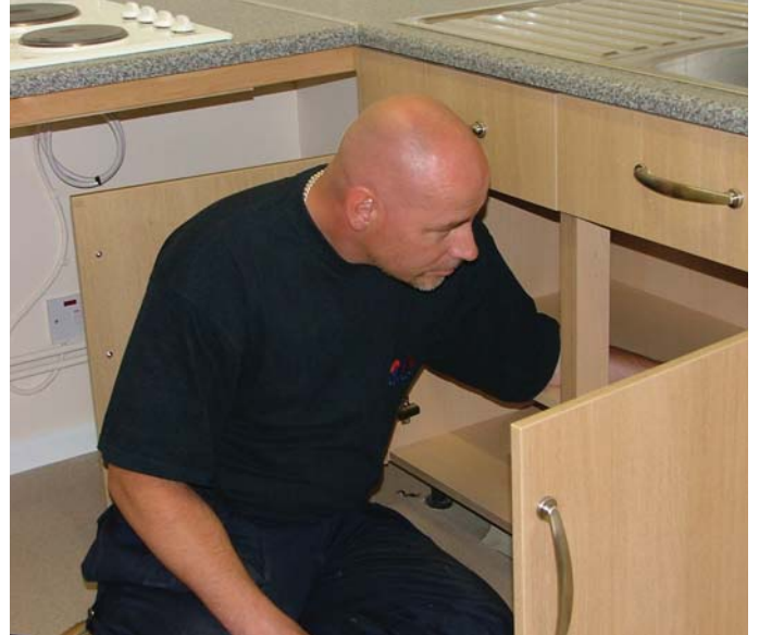
A Mountjoy contractor fits a new kitchen on the Isle of Wight. We reselected the company for one of our new partnering contracts.
